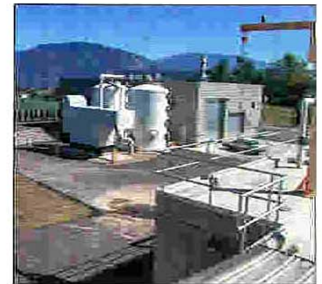
The Stage IIIB upgrade to the City of Salmon Arm's Water Pollution Control Centre includes multi-stage odour treatment.
