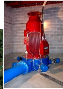
Powerhouse – Turbine, generator and inlet piping.†
