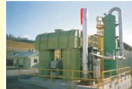
Recuperative Thermal Oxidation (RTO) Treatment for VOC Trans Mountain Pipeline Company Ltd.
