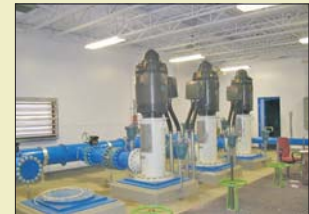
Fishtrap Creek Water Pump Station (Collector Well Below) City of Prince George, B.C.
