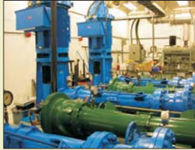
River Heights Water Pump Station City of Coquitlam, B.C.
