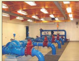
East Aldergrove Booster Pump Station Township of Langley, B.C.
