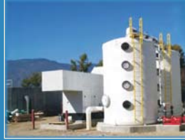
Bioscrubber and Ozone Contact Tanks
