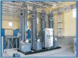
ATAD 4-stage Scrubber
