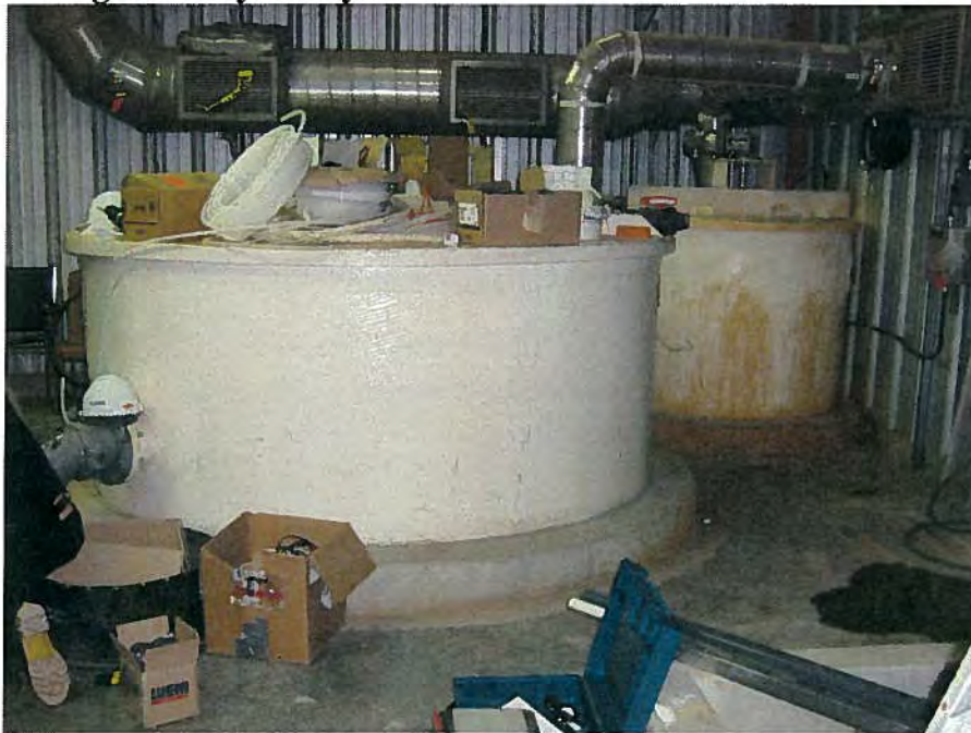
Figure 2 - Cylindrical Centrate storage tanks with conical bottom (in lower floor), taken during assembly of Crystallizer
