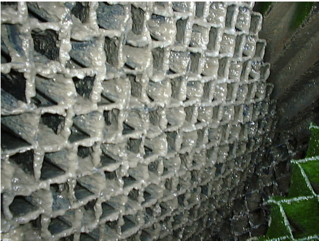
Figure 4 Photograph of Nuisance Slime Growth on Trickling Filter Media
