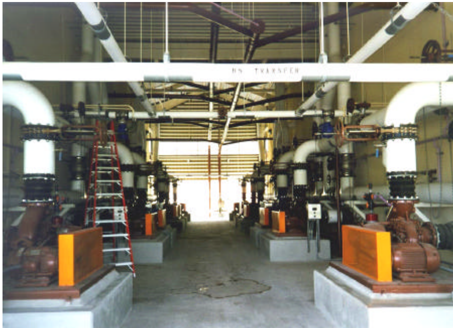
Figure 9 - City of Sunrise, Florida, Sawgrass WWTP ATAD Pump Gallery
