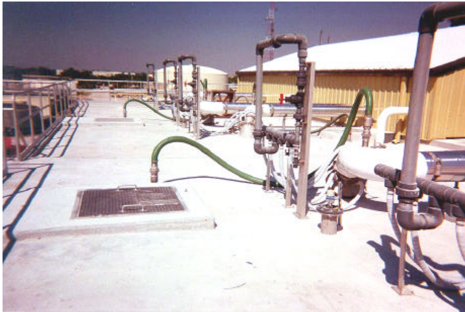
Figure 11 - City of Sunrise, Florida, Sawgrass WWTP ATAD Venturi Aerator Nozzles
