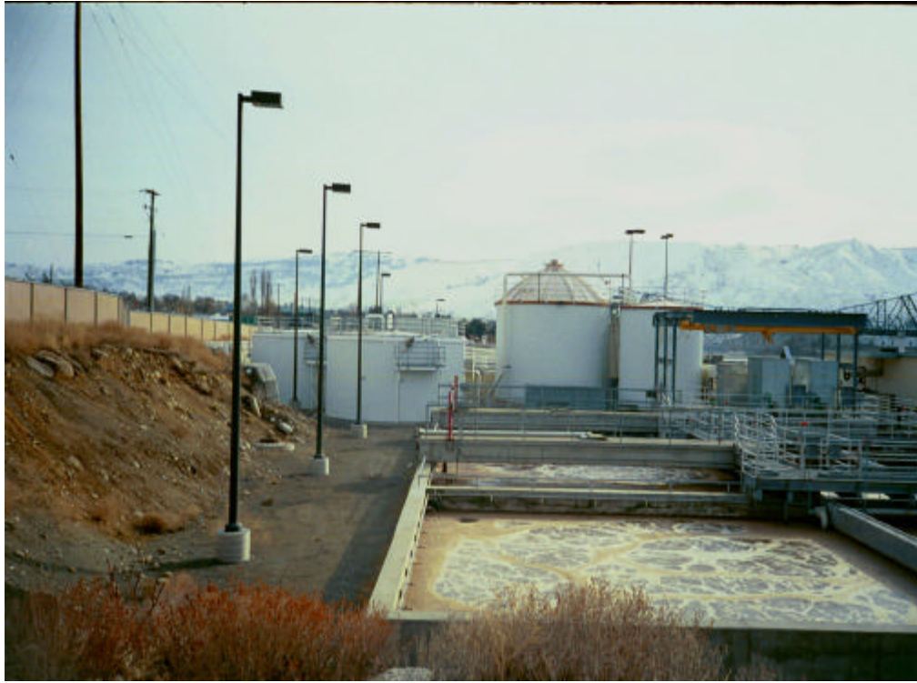
Figure 19 - Douglas County WWTP, ATAD Digesters in left background, pre and post holding tanks in center-right background.
