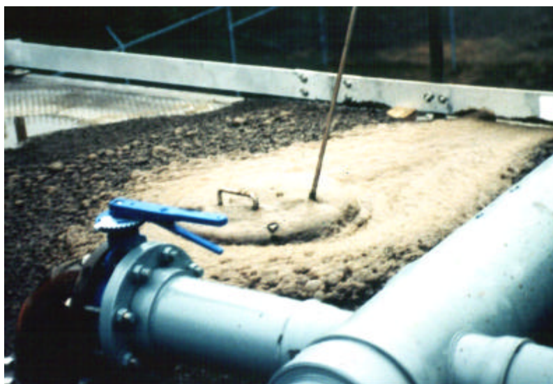
Figure 3 - Foam Flooding on Small ATAD Reactor without Foam Protection Systems
