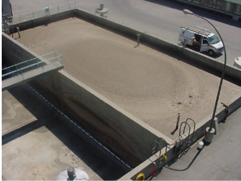
Figure 6 - NW Langley, B.C. WWTP Aerobic Digestion
