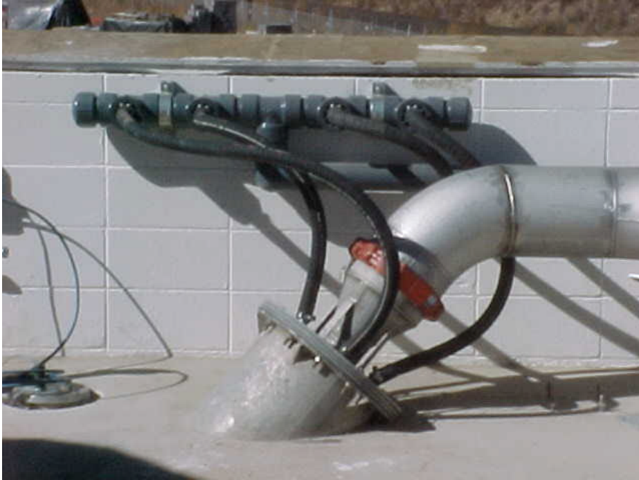
Figure 13 – Edwards, CO, WWTP ATAD Venturi Aerator Nozzle Mixer
