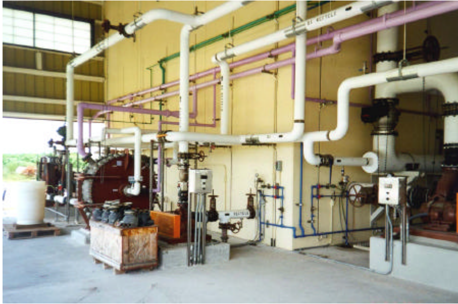
Figure 10 - City of Sunrise, Florida, Sawgrass WWTP ATAD Heat Exchanger
