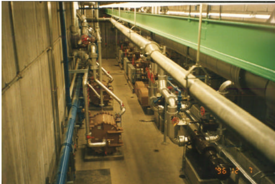
Figure 14 – Avon, CO, WWTP ATAD Pump Gallery
