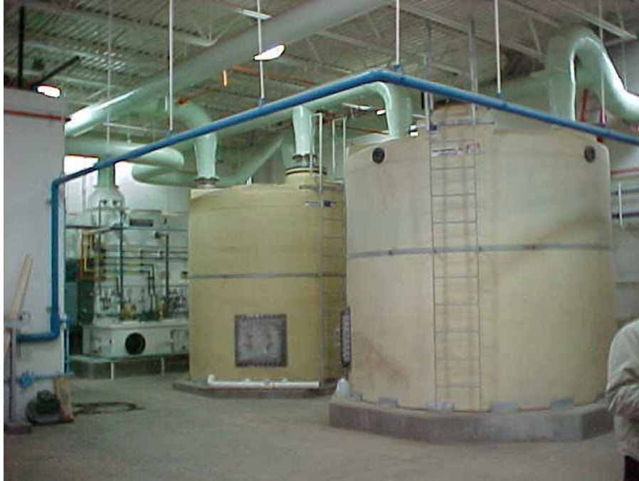
Figure 15 – Edwards, CO, Odor Control, NTF, Ozone Wet Chemical Scrubber
