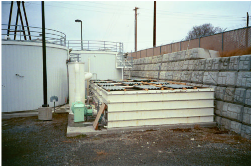
Figure 20 - Douglas County WWTP Odor Collection and Treatment using water scrubber and soil-bark filter bed.
